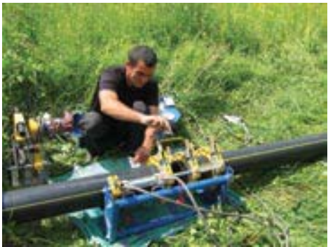
Setting up the connection and distribution of water systems to the village.
