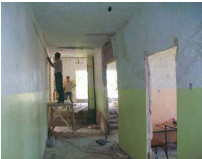
Major work is being done to rebuild the Noyemberyan Hospital in Tavush.
