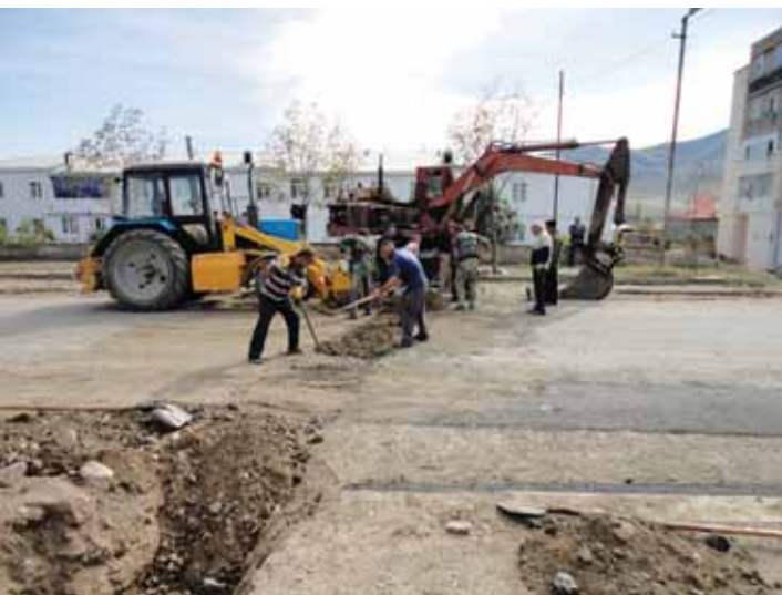
A new internal distribution network is being constructed to bring potable water to Karmir Shuka village in Martuni, where 200 villages await clean drinking water.
