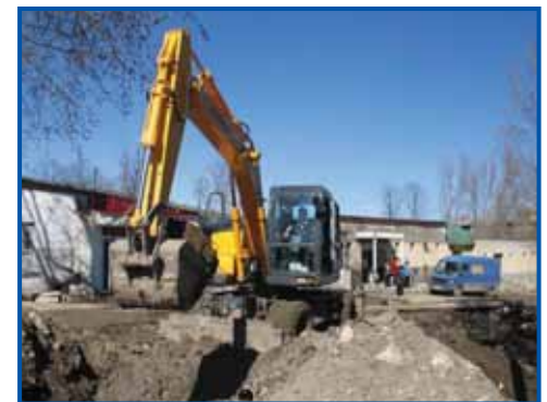
Previous Shushi utility infrastructure, such as sewers and gutters, were dysfunctional and dangerous.
