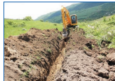
This trench will bring water down from the mountain to the village below.
