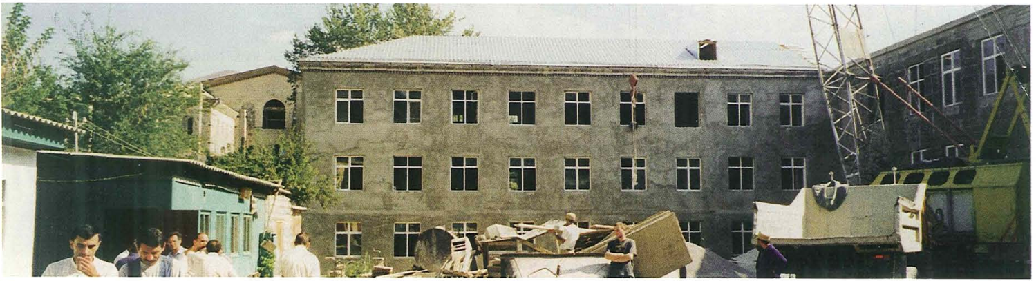
The reconstructed Vanadzor School, alma mater of many of Armenia's most notable artists, scientists, politicians and writers, will be a modern educational institution and a community-based enterprise to enhance learning and build sustainability.
