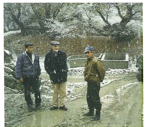
Kevork Toroyan, Armenia Fund USA Vice Chairman, at the construction site for the North-South Highway.
