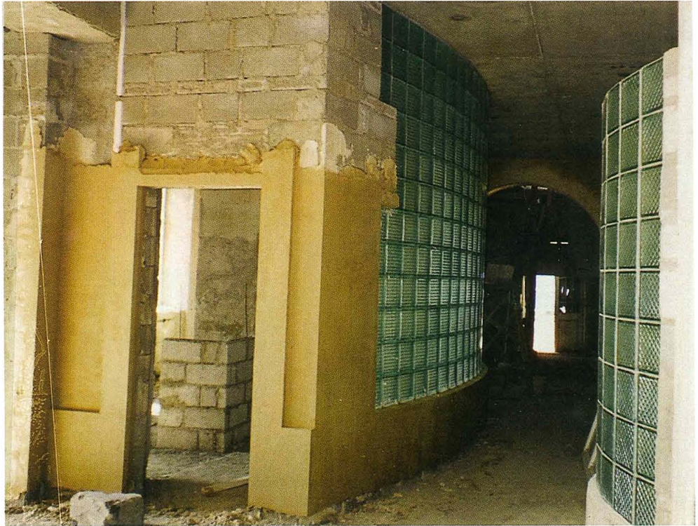
Thanks to generous donations and speedy workmanship, the construction of the Vanadzor School is ahead of schedule.
